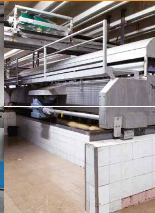
Malt house turner with 14 drives and traveling drive
